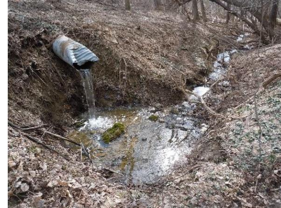
Drain Tile Discharge Pipe
