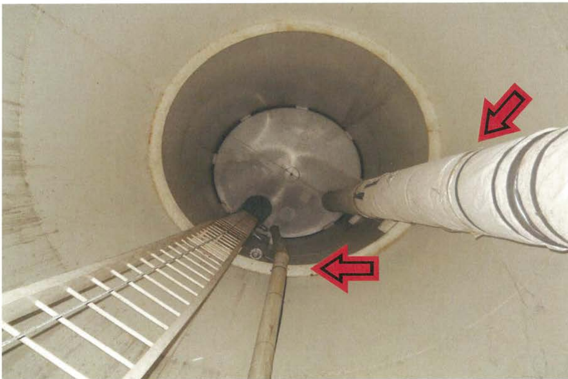
Photo shows the piping insulation which appears to be in adequate condition to prevent pipes from freezing.
