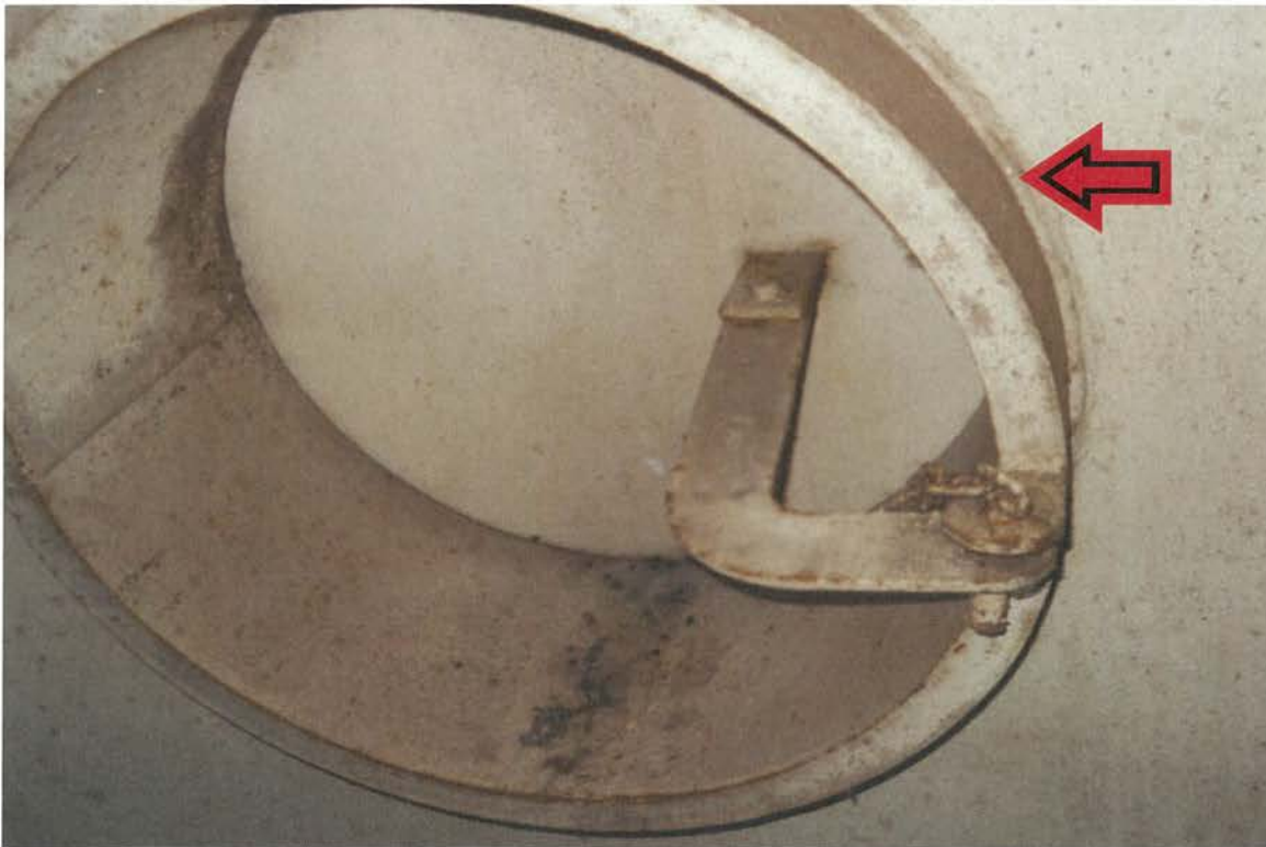
Photos show the painters hatch which appears to be in good condition.
