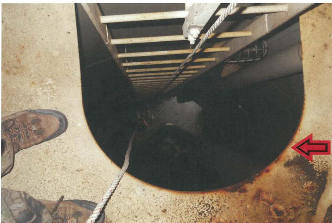
Photo shows the condensate platform, which appears to be in good condition. We recommend installing a drain tied into the overflow pipe and a hinged grating over the opening to prevent a falling hazard.
